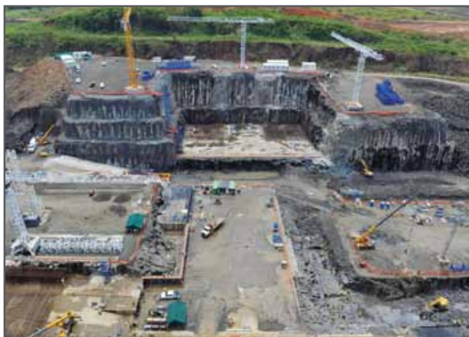
Work in the area of one of the Third Set of Locks gate recesses on the Atlantic side
